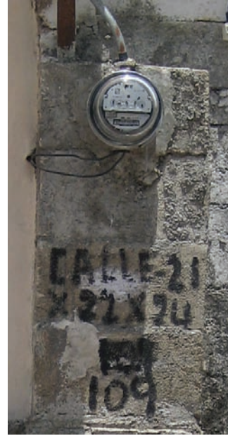
Utility meter in Mexico
