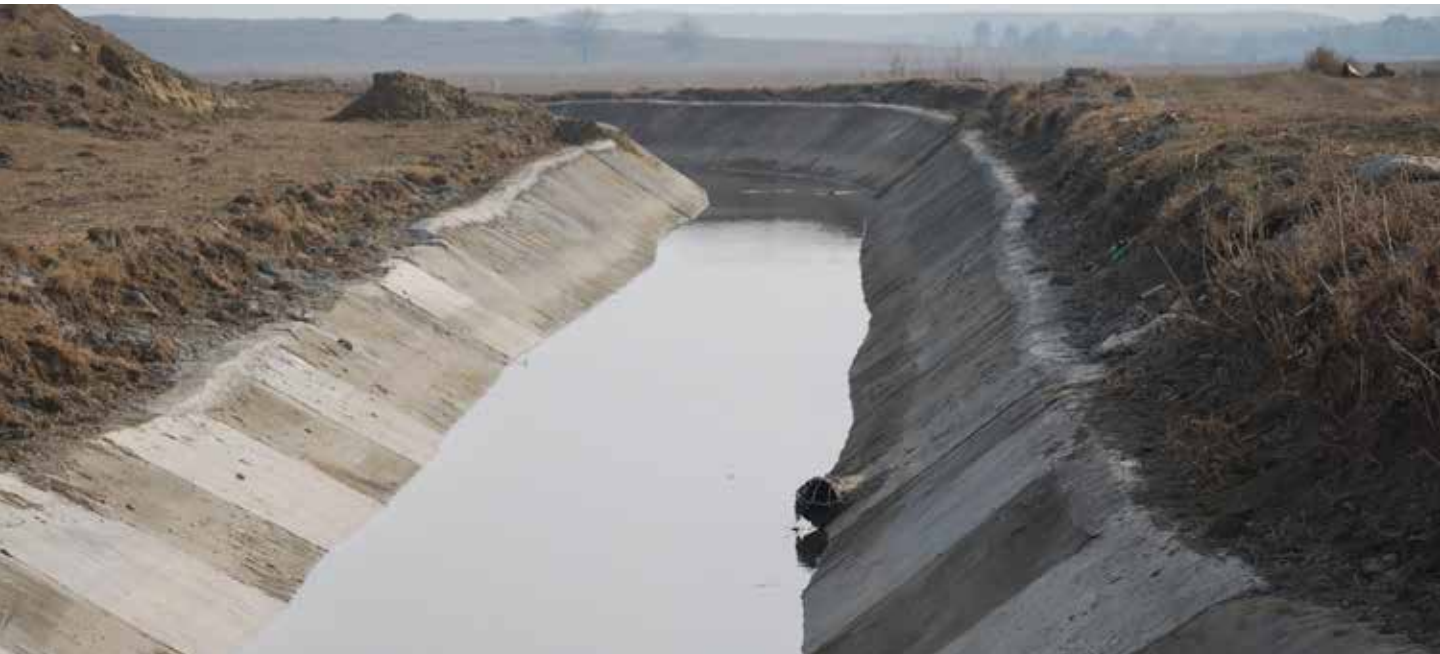
Irrigation canal in Azerbaijan built following clearance by ANAMA the Azerbaijan National Agency for Mine Action. © Charles Downs
