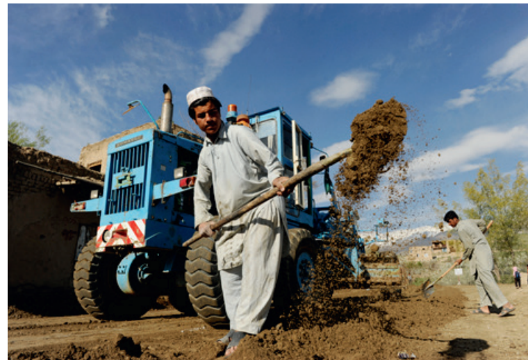
Young Afghan takes part in road-building works supported by UNDP’s National Area -Based Development Program in Kabul province, Afghanistan. © UNDP Afghanistan
