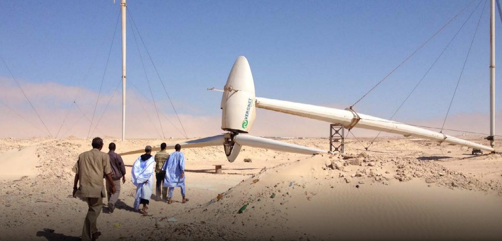
A UNDP Mauritania team visits a wind-power plant at Nouadhibou to examine a downed turbine. UNDP supports the Government of Mauritania in promoting clean and renewable energy, having helped prepare an assessment that calls for increasing power generation, developing the power grid, and boosting the role of renewable energy in the national-energy mix.
