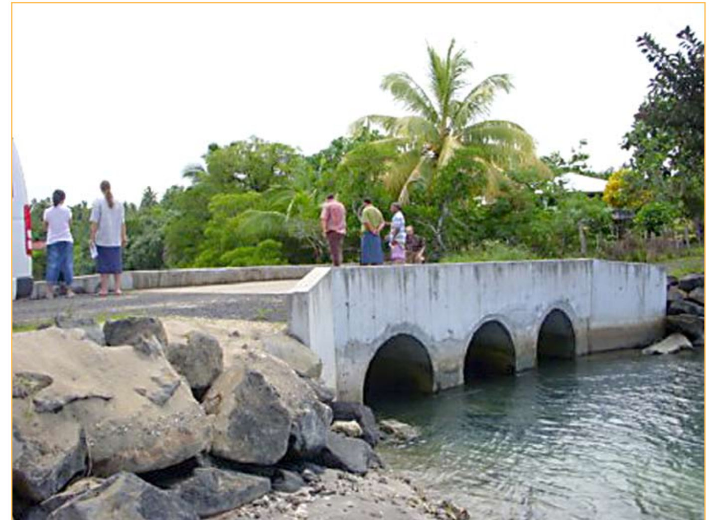
Box culverts help water flow more easily during severe flooding.
