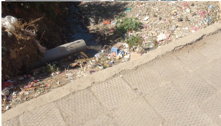
Conflict case of Jebelah hospital sewerage system
