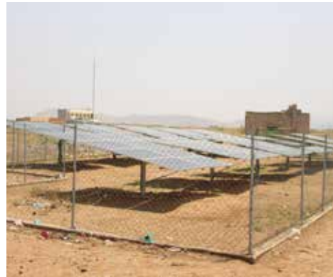
Al-Dhiaibi water project, that conducted by UNFICEF, Bajil District, Hodeidah (Photo: AFCAR)
