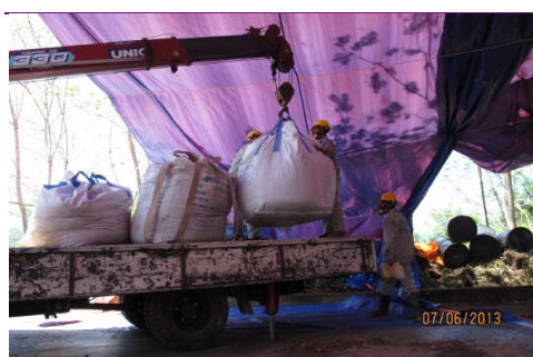
Figure 4.6 Using a crane truck or the backhoe the big bags were moved onto pallets in zone 2
