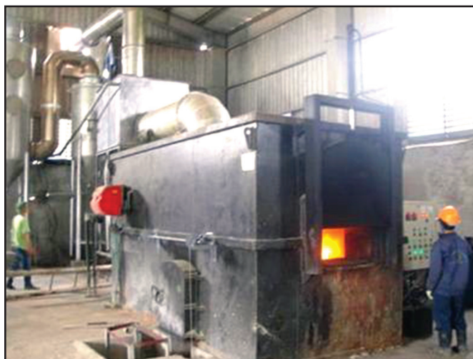
Figure II.10: A hazardous waste incinerator made in Vietnam
