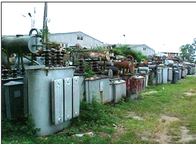
Figure II. 3: Stored transformers after use
