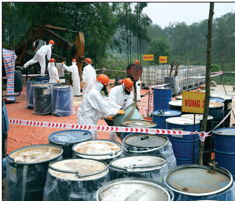
Figure II.11: Treatment of POP pesticides stockpiles
