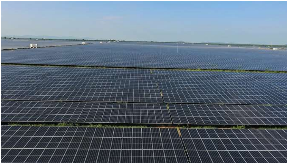
Figure 5. Solar power panels in Xuan Thien – Ea Sup 11
