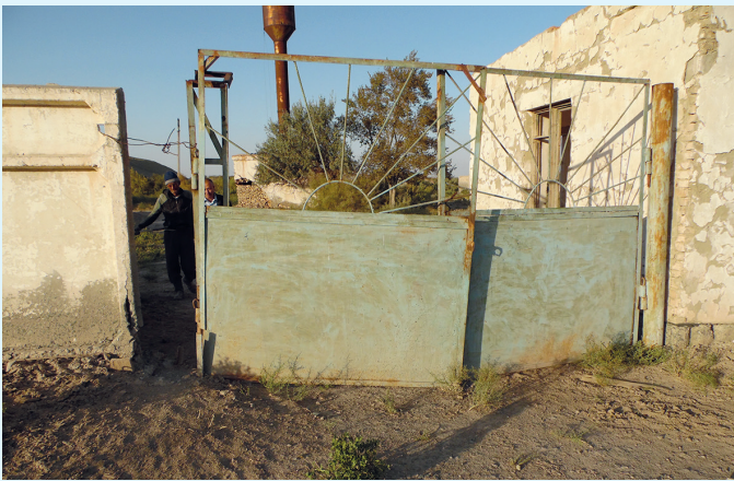
Pic.3. Water treatment plant, "Taza-Konys" community, 2019.
