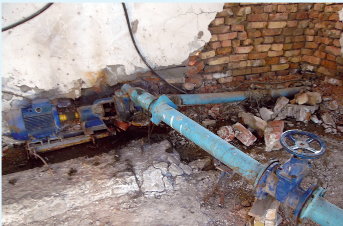
Pic.5. Water pipelines at "Taza-Konys" community were not functioning, 2019.
