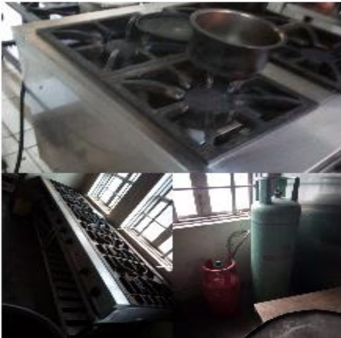
Institutional LPG gas stove with multiple cook points
