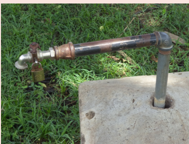
Tap Kalisizo Hospital-Rakai
