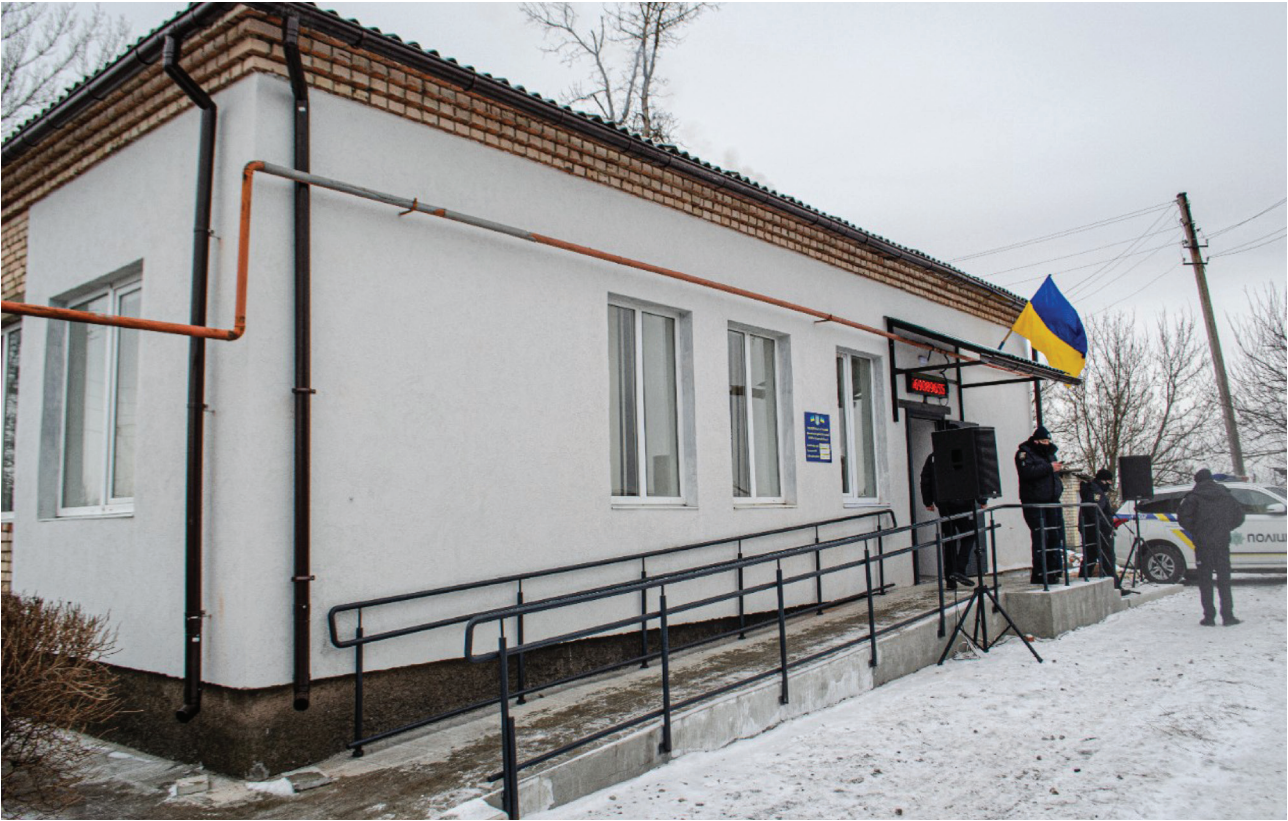
UNDP under the United Nations Recovery and Peacebuilding Programme renovated a police station in the Triokhizbenka community, Luhansk Oblast, which is located 2 kilometers from the conflict's 'contact line' in eastern Ukraine. The work to renovate the police station was carried out with the financial support of the governments of Denmark, Sweden and Switzerland. Photo: Vitaliy Shevelev / UNDP Ukraine
