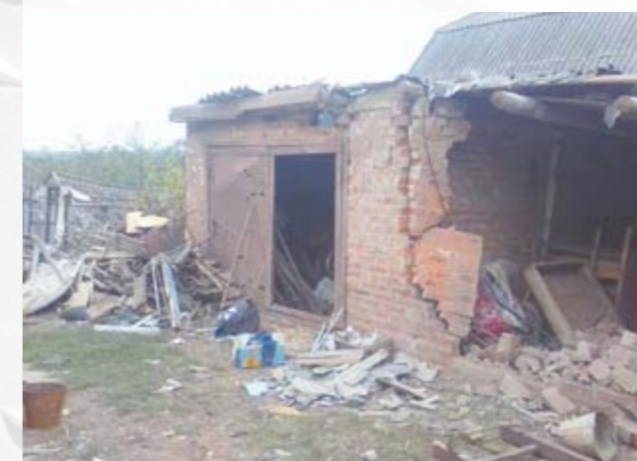
Damaged household in Verkhnyotoretsk 2
