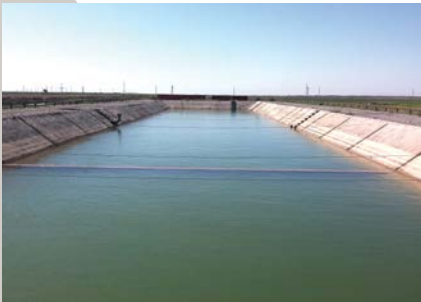
A water desilting tank designed to filter water from the channel before it reaches the field for irrigation at the UNDP-supported research demonstration site in Geokdepe.
