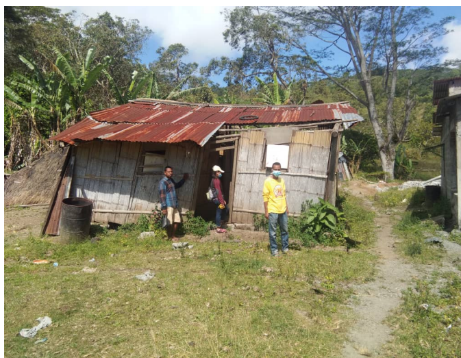
Figure 36: A semi-permanent type house damaged
