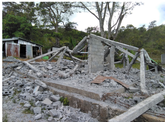
Figure 34: A damaged CGI sheet house
