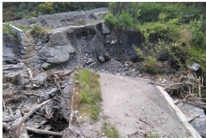
Figure 49: Bridge damaged by Easter floods, Baucau
