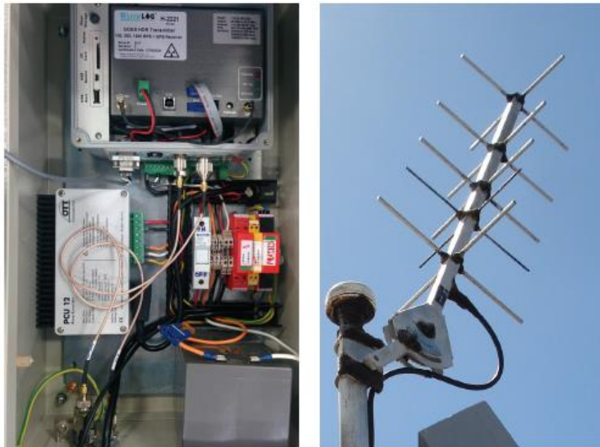
Figure 21. Example of the internal components of the radar gauge control unit (left) which included data logger and connections to telemetry instruments. The radar gauge control unity is connected via cable to the telemetry systems antenna (right).
