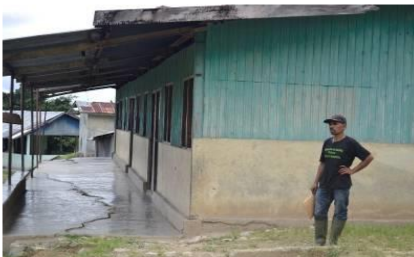
Figure 12 – Damage to primary school caused by erosion and slumping. Abo Suco, Seiçal River Catchment
