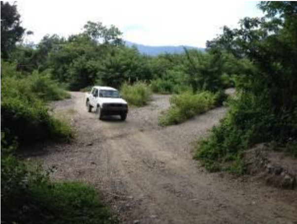
Figure 42 – Flash floods cause erosion and deposit sediment, damaging roads and other infrastructure. Guiço Suco, Lois River Catchment
