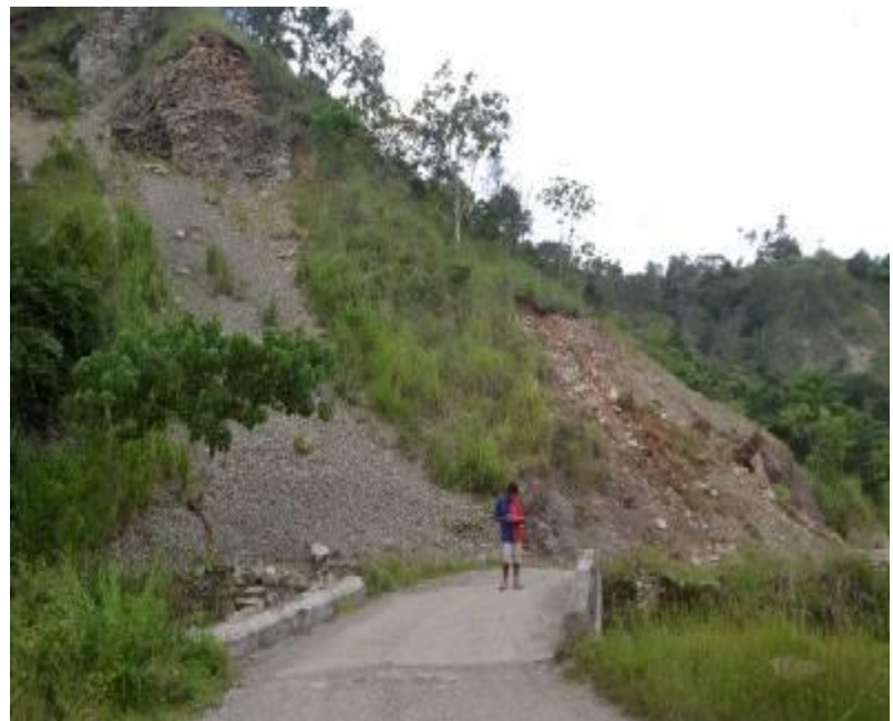
Figure 8 – Landslide closing road and threatening bridge, caused by steep slope, unconsolidated rock, thin vegetation. Baguia Suco, Boro Uai Catchment
