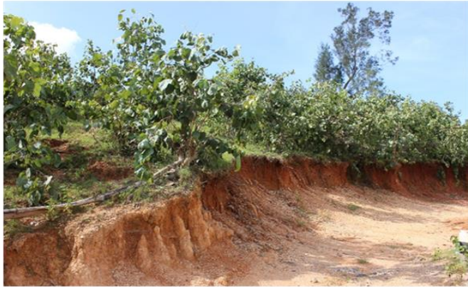
Figure 34. Road itself eroding away. Ulmera Suco, Comoro River Catchment
