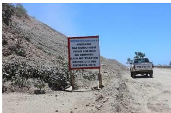
Figure 33 – Recently re-opened road after landslide clean-up. Ulmera Suco, Comluli Aggregate
