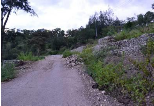
Figure 9 – Evidence of flash-floods, landslides and erosion, and engineering efforts to protect road.
