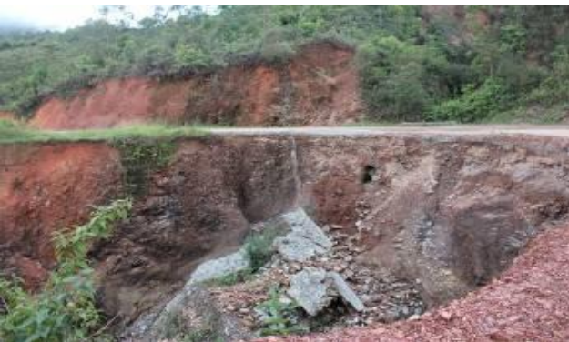
Figure 19 – Part of main road from Letefoho to Gleno, removed by landslide. Humboe Suco, Lois
