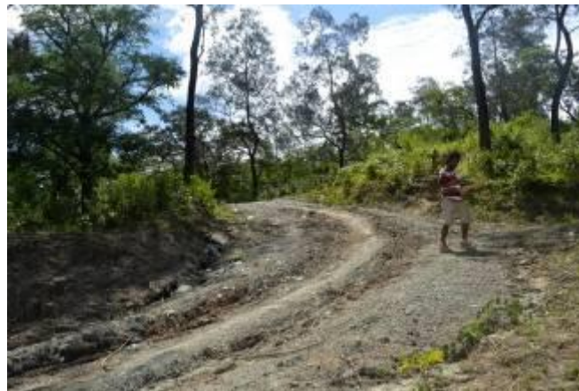
Figure 15 – Road in poor condition in high-risk area for erosion. Ossouala Suco, upper Vemasse River Catchment
