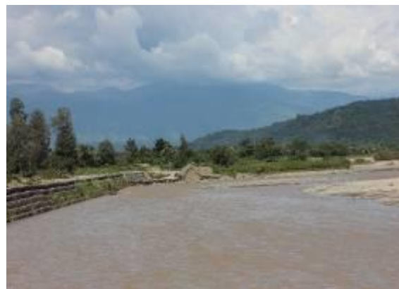
Figure 44 – Gabions protect farmland, irrigation systems, houses, schools and health clinics from river erosion. Vatuboro Suco, Lois River Catchment
