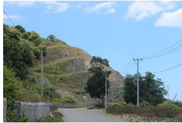
Figure 39 – Terracing to strengthen and reduce steepness of slope and thus lessen threat to road from landslides and erosion. Gualeur Suco, Kaikasa
