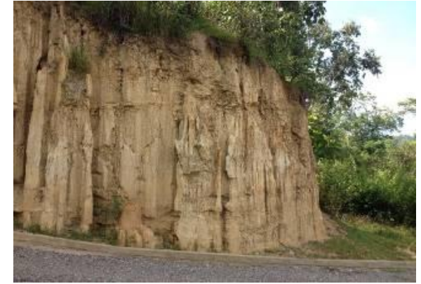
Figure 36 – Sparse vegetation on highly erodible soils. Near Lebulua, Ulmera Suco, Comoro
