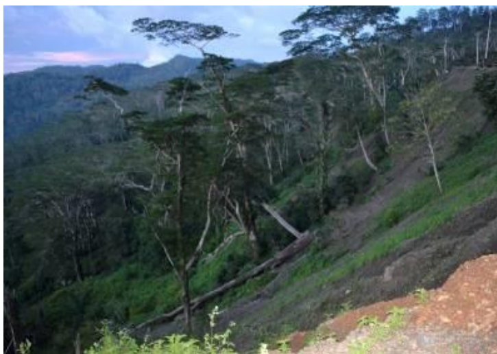
Figure 27 –Landslide triggered by road construction on sparsely-vegetated moderate slope. Ailelo Suco, Lois River Catchment
