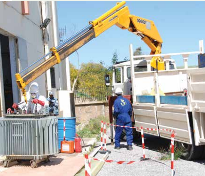
PCB-containing transformers are transported for disposal. Photo by UNDP Morocco
