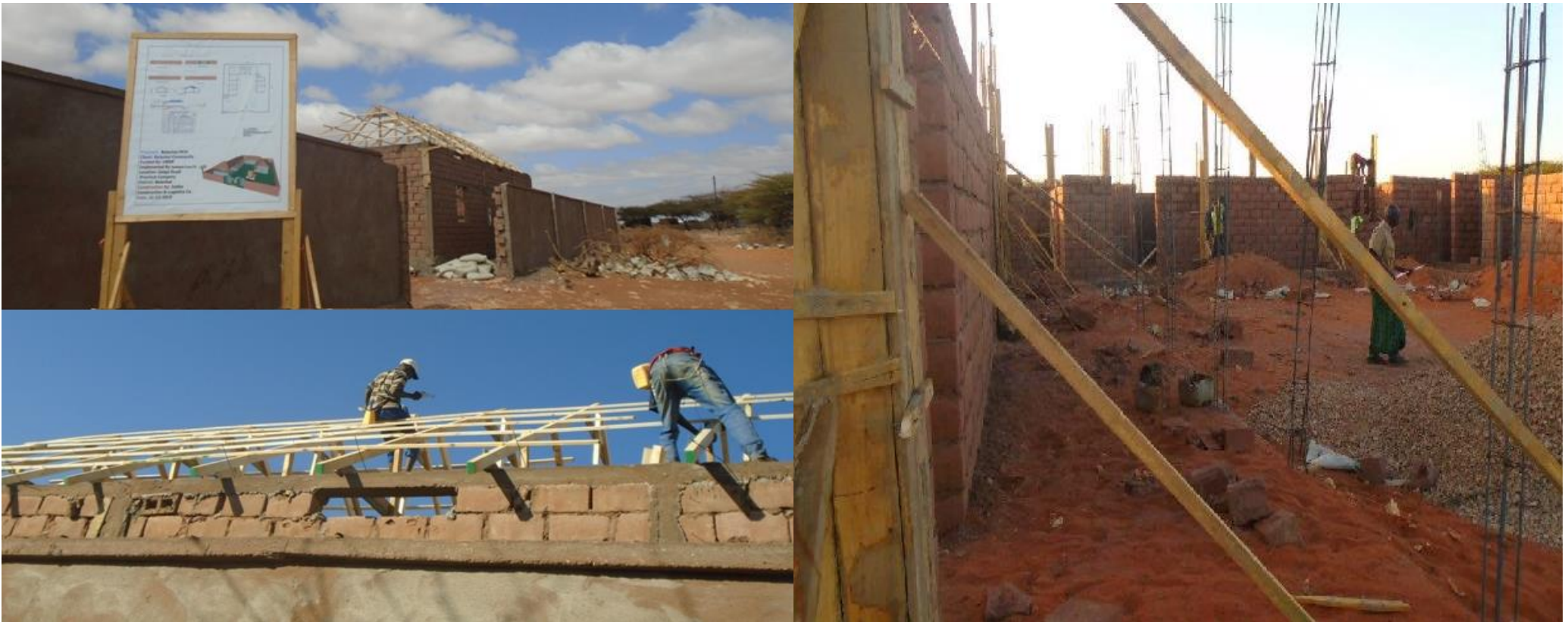
Photo: Construction work of Mother and Child Health Facility (MCH) in Balanbale
