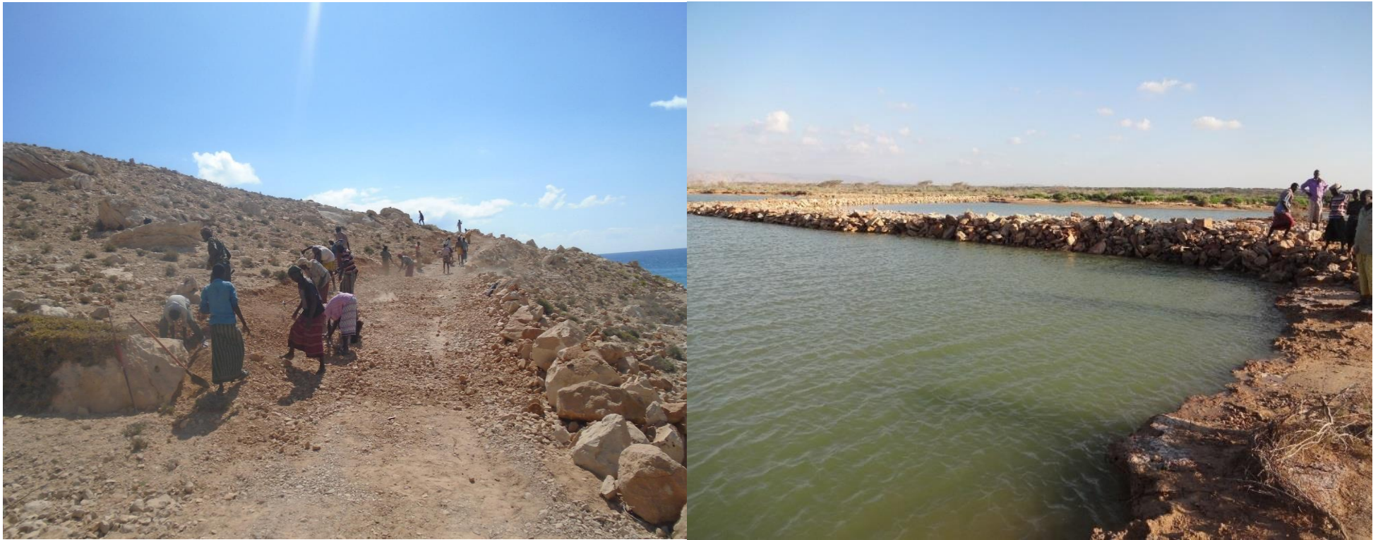
Photo: Rehabilitation of Lafagorayo road and rehabilitation of road that divides the Alula.
