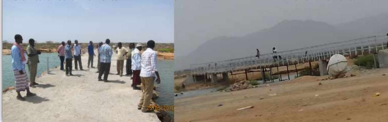
PHOTO 2: CONSTRUCTION WORK OF CULVERT BETWEEN ALULA AND BARGALE AND THE REHABILITATION OF HABO IRISH CULVERT
