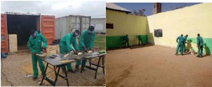
UNIDO plastering and painting skills training at the Baidoa Central Prison. Containerized training platform for woodworking (beehive box making)
