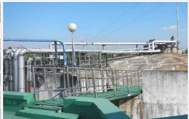
Bio-digestion pipe located in the Nanji Sewage Treatment Center
