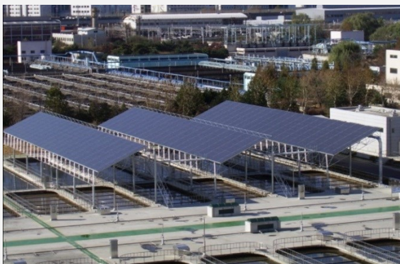
Photovoltaic power plant in the Jungnang Sewage Treatment Center
