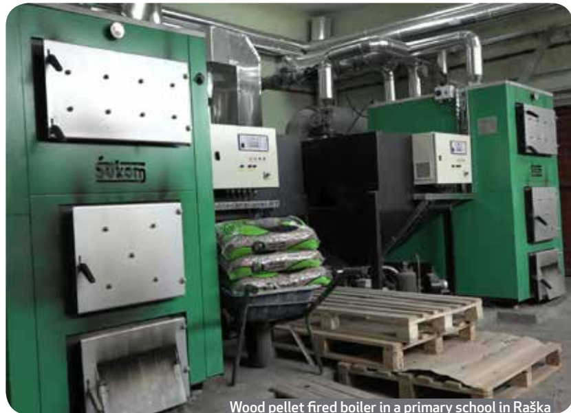
Wood pellet fired boiler in a primary school in Raška
