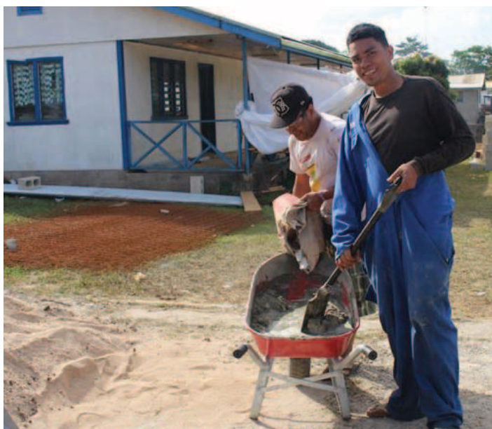
Private sector businesses in Tonga are assisting Mu'a residents to build risk-resilient community halls. (Photo: MORDIT T)
