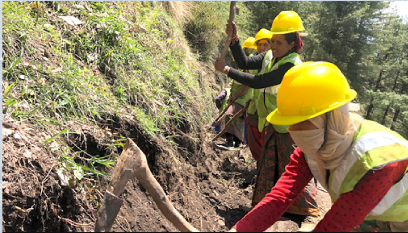
Community User Group of Bhulbhule Bhada Drinking Water Project, Jumla engaged in digging the pipeline
