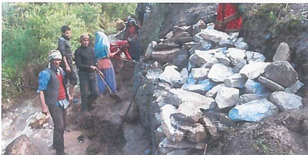
Picture 3: Community people working for gabion wall at Malikabota, Ghattekhola VDC, Jumla district
