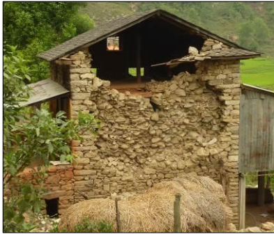
(a) Delamination and bulging of wall wythe, 2015 Gorkha earthquake, Nepal
