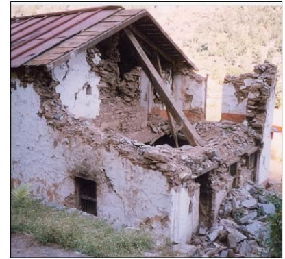
(f) Roof collapse due to absence of wall-roof connections, 1999 Chamoli earthquake, India
