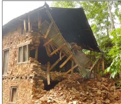
(b) Out-of-plane collapse of wall led to collapse of roof and floor, 2015 Gorkha earthquake, Nepal
