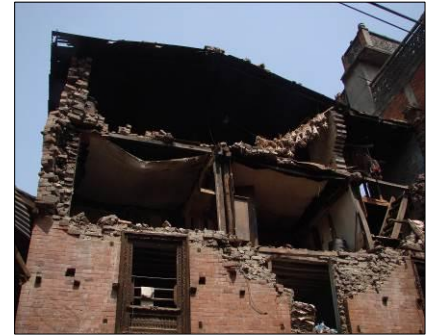
(c) Out-of-plane collapse of walls, destruction of top storey, 2015 Gorkha earthquake, Nepal
