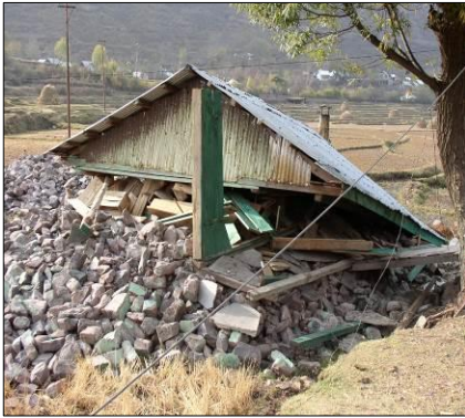
(d) Destruction of a house, 2005 Kashmir earthquake, Pakistan
