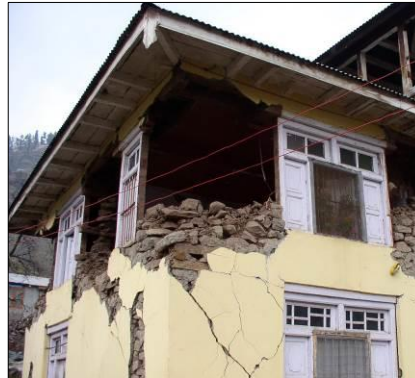
(e) In-plane wall and corner damage, 2005 Kashmir earthquake, Pakistan
