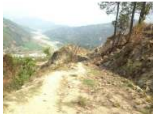
Slope failure and gulley erosion
