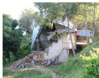
Figure 2.4 Collapsed structure (Source: CoRD)
