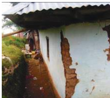
Figure 2.17 Corner damage during Eastern Nepal Earthquake, 2011 (Source: CoRD)
