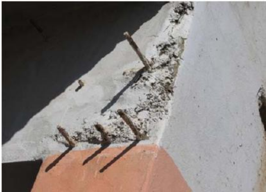
Rebar exposed at beam ends
