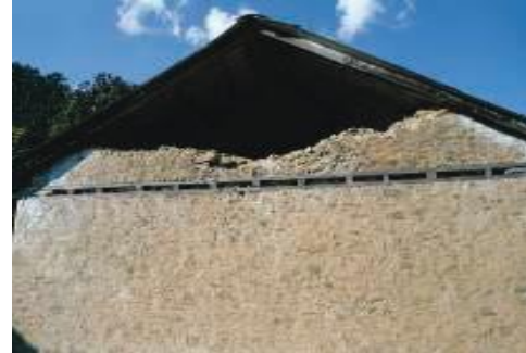
Figure 2.10 Gable end wall mid-height collapse (Sinam, Eastern Nepal Earthquake, September 1st, 2011)
