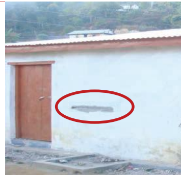
Figure 2.14 Mid-height Crack (Photo: CoRD)
