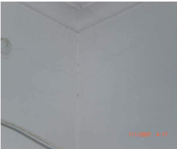
Figure B-19: Crack at wall
