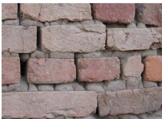
Void between masonry units
