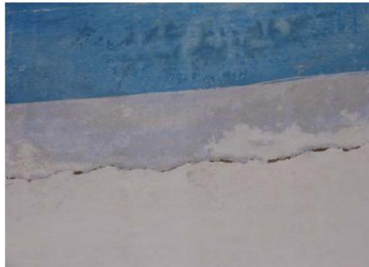
Cracks at slab & wall connection
