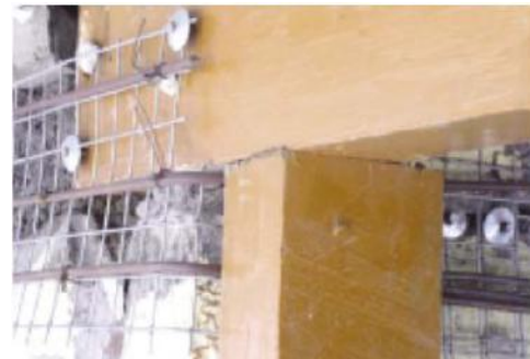
Figure A- 12: continuity at corner behind wood post obstruction
