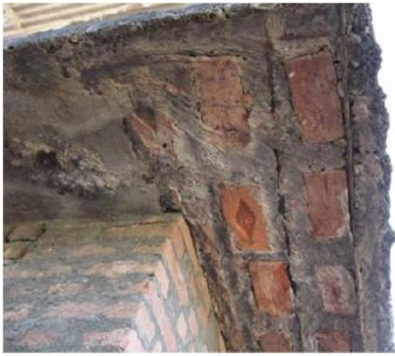
Rebar exposed in RBC slab
