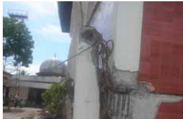
Soft Ground Storey
