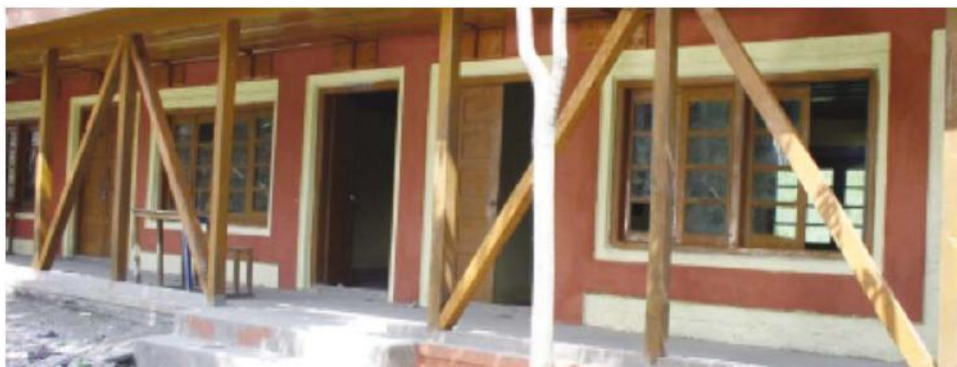
Figure A- 20: Retrofitted building with belts, roof anchoring and diagonal timber bracings
