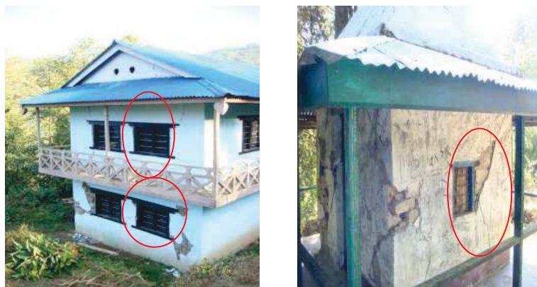
Figure 2.24 Some examples of Cracks at opening
