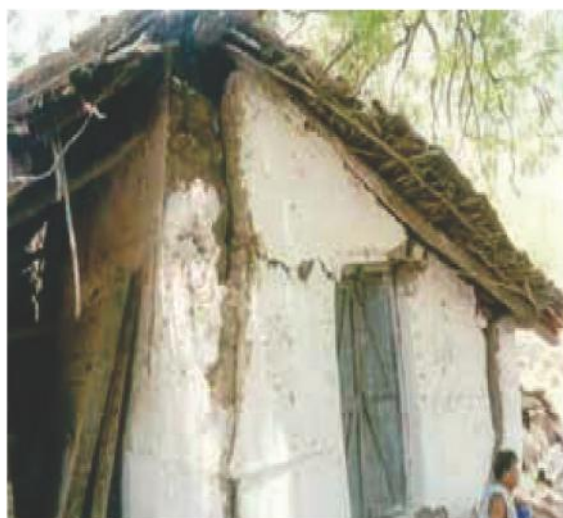
Figure 2.19 Vertical cracking and separation of adobe walls after the 1997 Jabalpur, India earthquake (Source: Kumar 2002)
