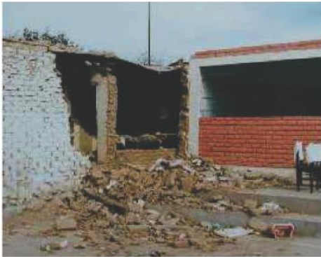
Figure 2.7 Out-of-plane wall collapse – 1996 Nazca earthquake, Peru (Source: Report #52 in EERI/ IAEE World Housing Encyclopedia)
