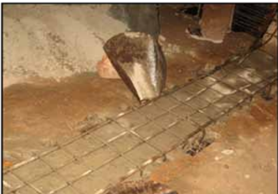
Figure 6.14 Beam Jacket (Source: MRB & Associates)
