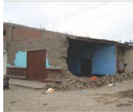
Figure 2.8 Out-of-plane wall collapse after the 2007 Pisco, Peru earthquake (Photo: M. Blondet)
