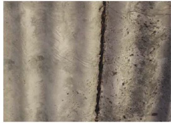
Rebar exposed in RCC slab
