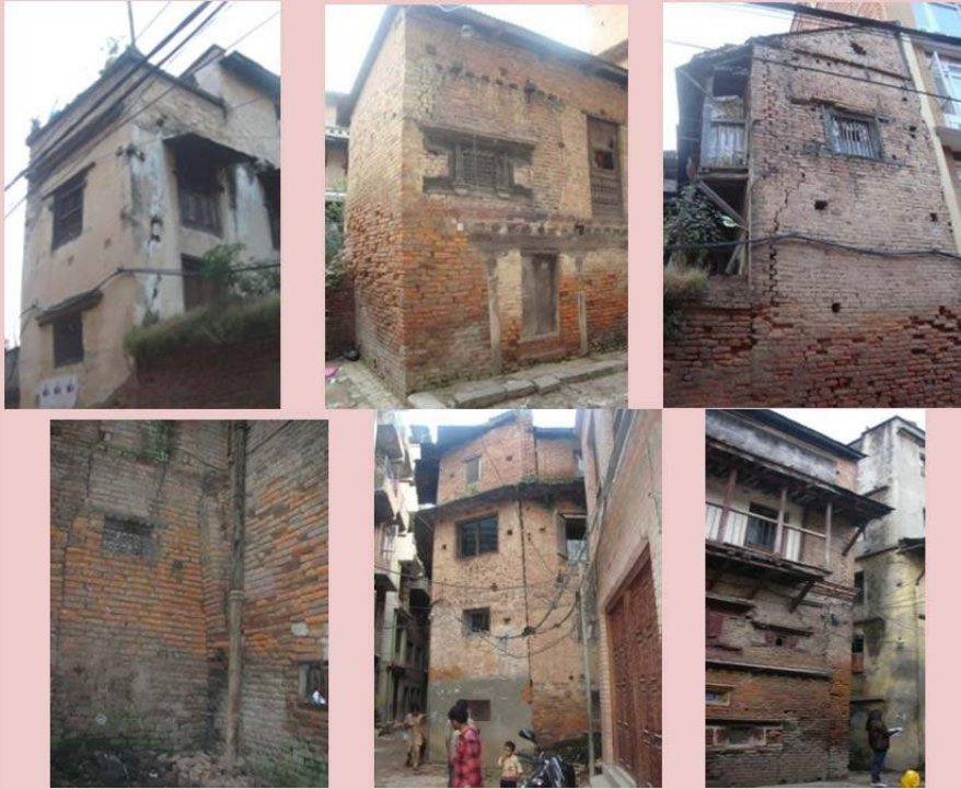
Cracks seen at corners in old buildings in Lalitpur, Nepal Photo: Ar. Anjali Manandbar
