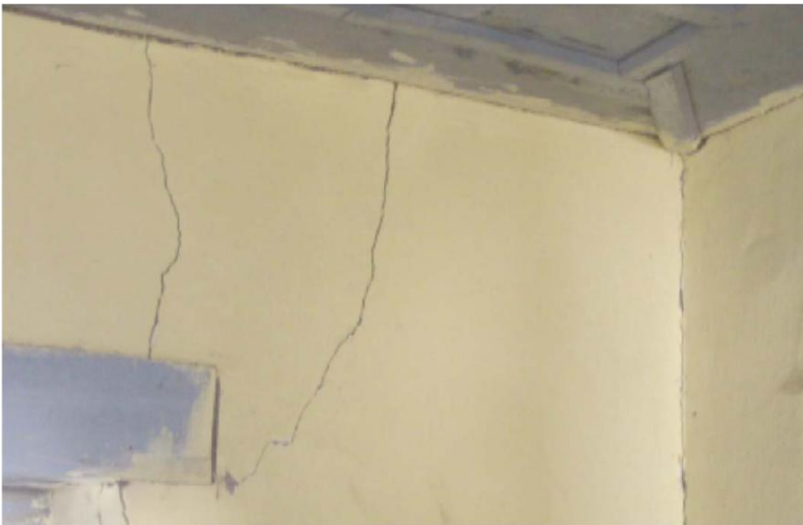
Figure A- 3: Typical cracking in corners and at corners of opening such as windows
