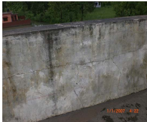
Figure B-20: Crack at Parapet wall
