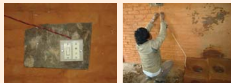
Switch box connected using electrical wire
