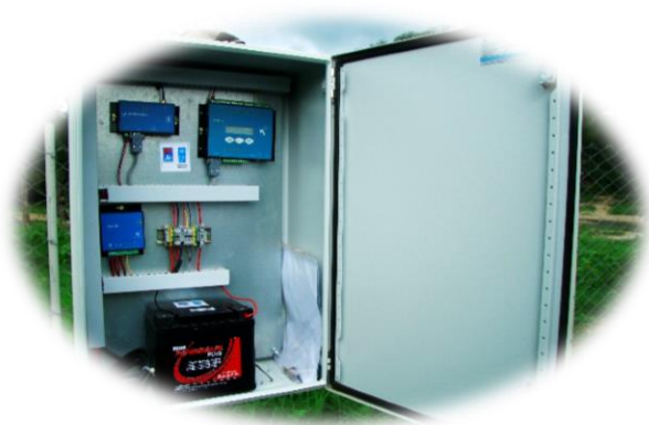
Community based Early Warning System, Riu-khola, Maadi, Chitwan
