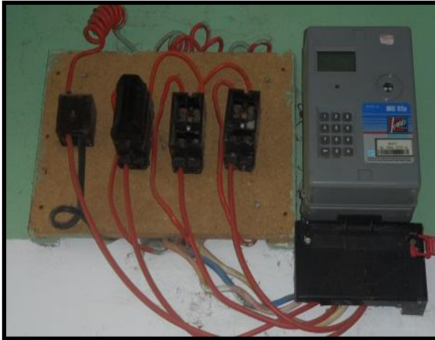
Distribution Board looped from the mains as a single phase
