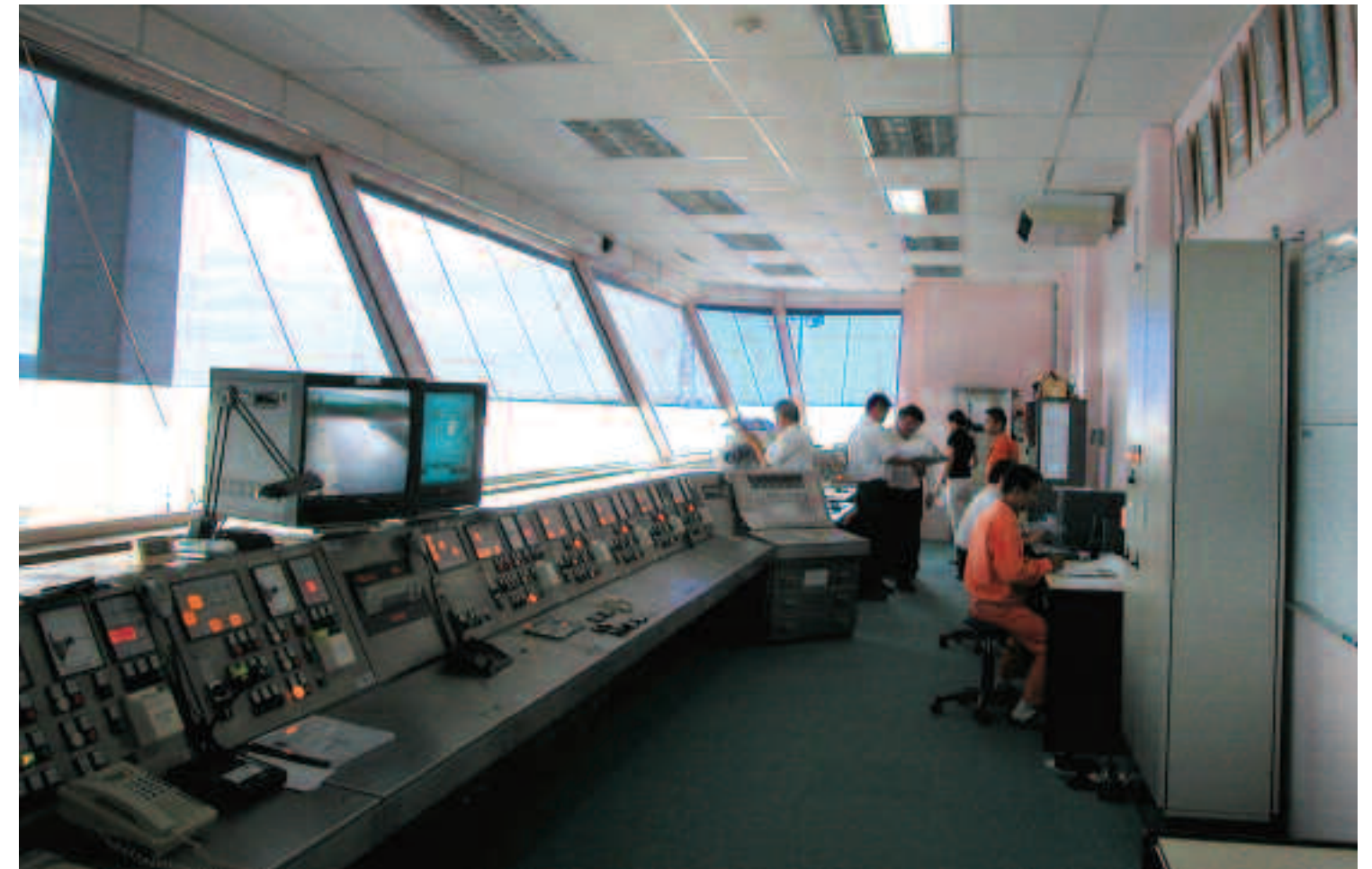
Kuching Barrage's control tower monitors rainfall sensors upstream, a flood warning system and the shiplock.
