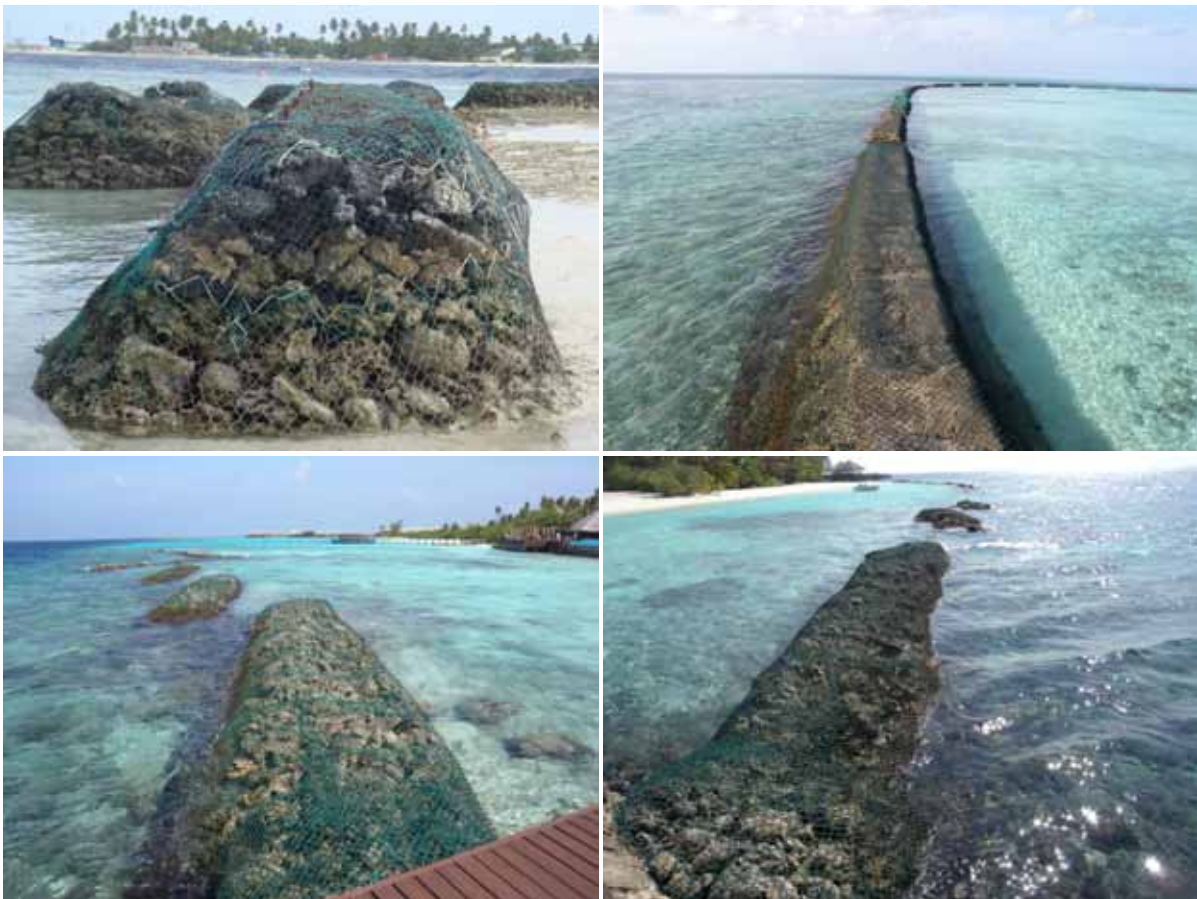
Figure 4.18: Generic fore-shore break water design – coral mound in (Clockwise from left) Dh. Vilureef, Lh. Komandoo and K. Boduhithi
