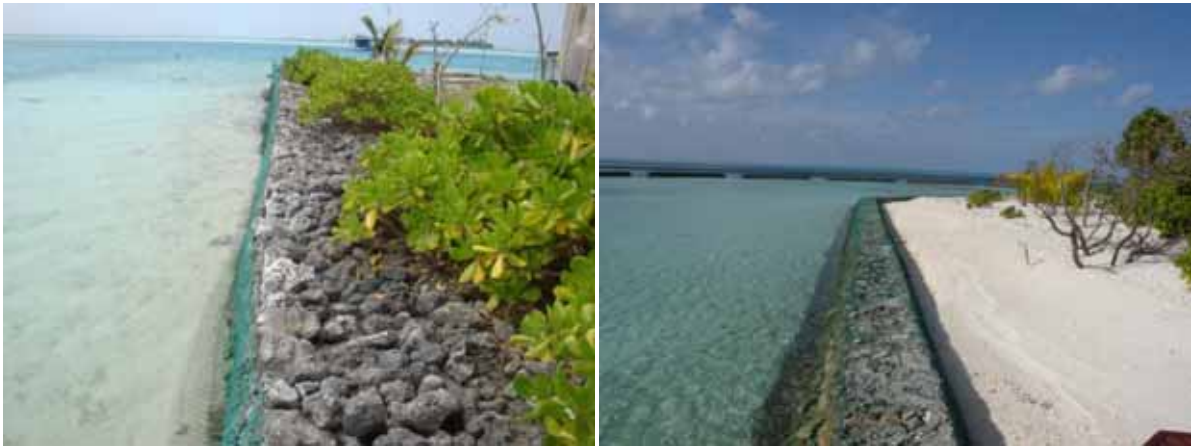
Figure 4.9: Examples of Sewall structures: unplastered sand cement bag seawall in M. Maduvvari and Sun Island Resort
