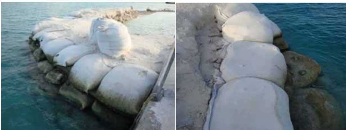
Figure 4.15: Examples of Sewall structures: Geo-bags in GDh Thinadhoo
