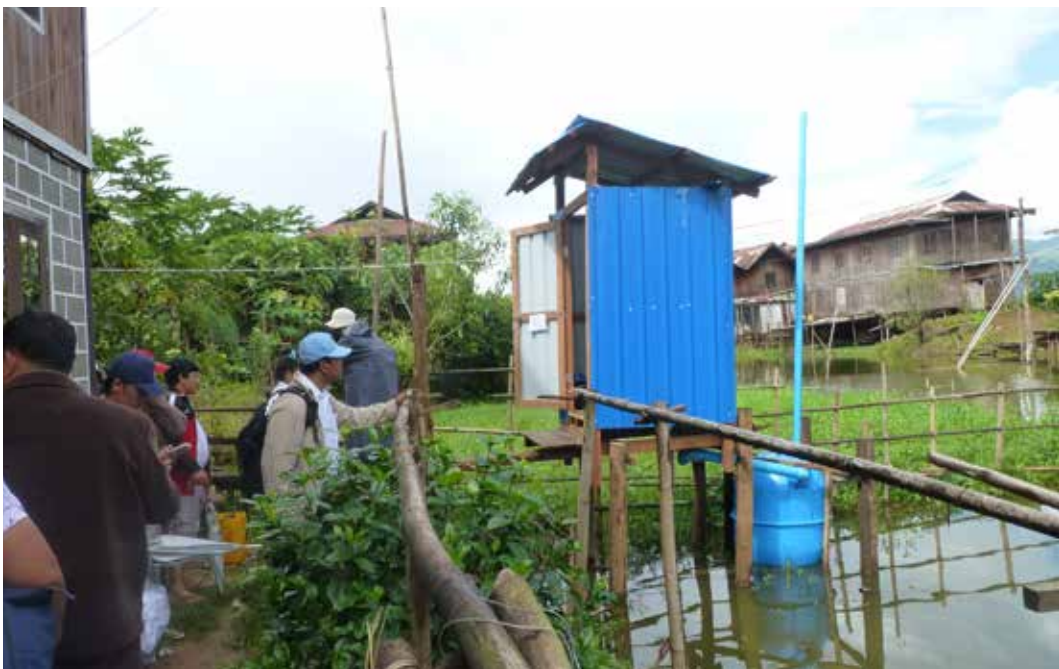
Bio-septic tank installed in Shan Ywar Le Pyin village, Nyaungshwe Township
