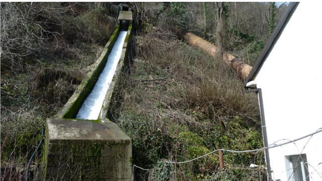
Figure 4: Penstock for the Rijeka Crnojevica SHPP
