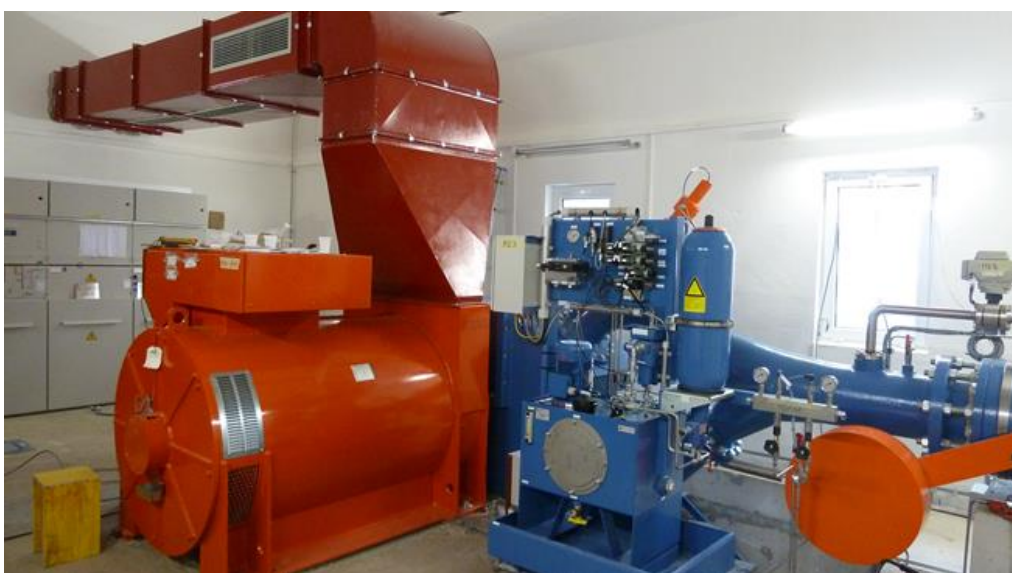
Figure 9: Newly Constructed Jezerstica SHPP Interior, Berane Municipality Turbine, Ventilation System, Generator, and Hydraulic Equipment
