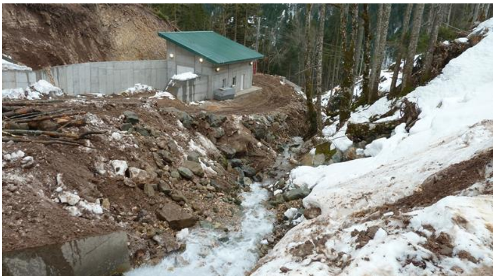
Figure 8: Newly Constructed Jezerstica SHPP, Berane Municipality
