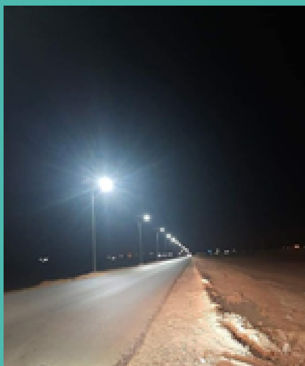
Solar streetlights already installed are working
