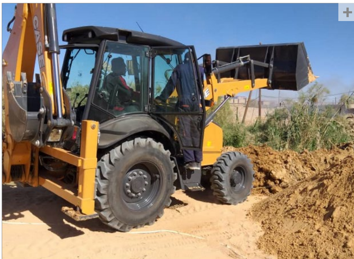
JAN 2020, GHAT (LIBYA). A backhoe loader is cleaning a water line in Ghat. Photo: ©UNDP Libya
