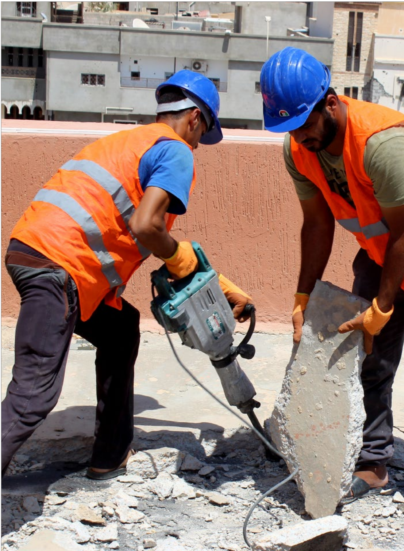
27 AUG 2018, SIRT, (LIBYA). Two workers are removing concrete on the roof of Al Fath school. The UNDP's Stabilization Facility for Libya renovated the educational institution and enabled 1,100 students to attend classes in better conditions. Photo©UNDP Libya/Abdeladeem Ajaj
