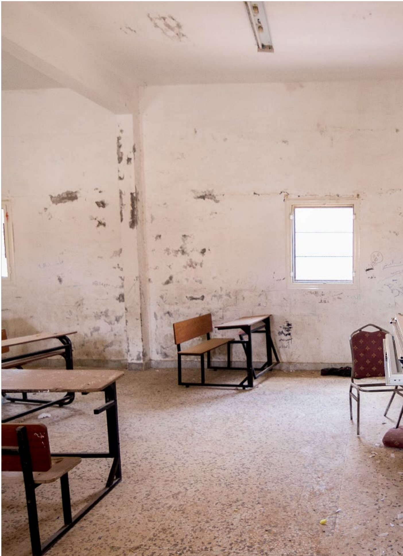
14 AUG 2018, TAJOURA, TRIPOLI, (LIBYA). Omar Almkhtar School, before the Stabilization Facility for Libya rehabilitated it. Photo: ©UNDP Libya/Malek Elmaghrebi
