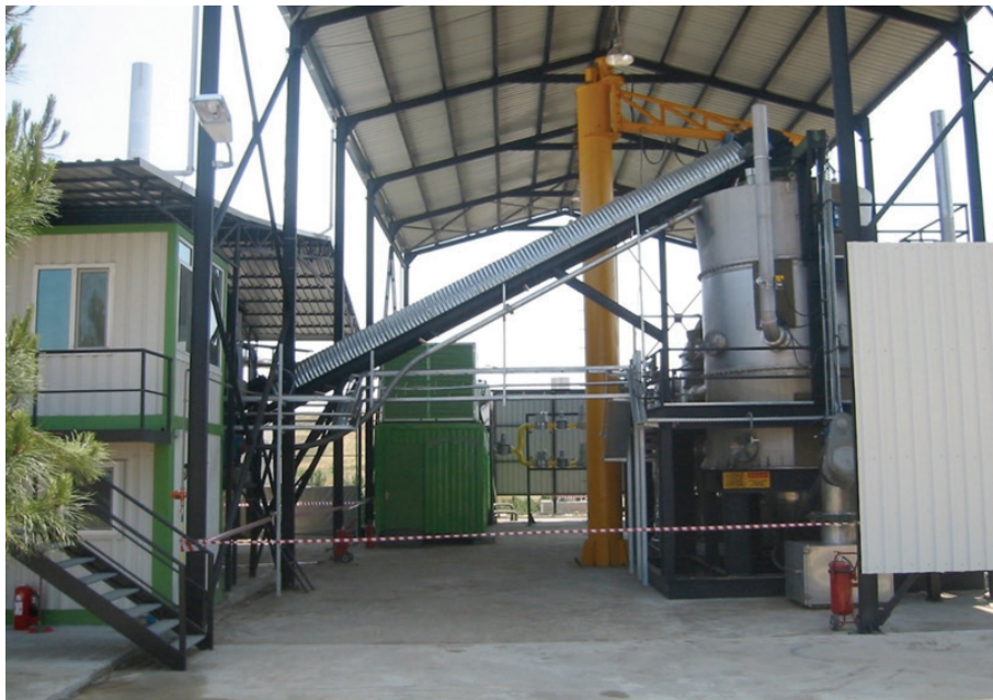
Figure 1.2: Gasifier and Syngas Engine
