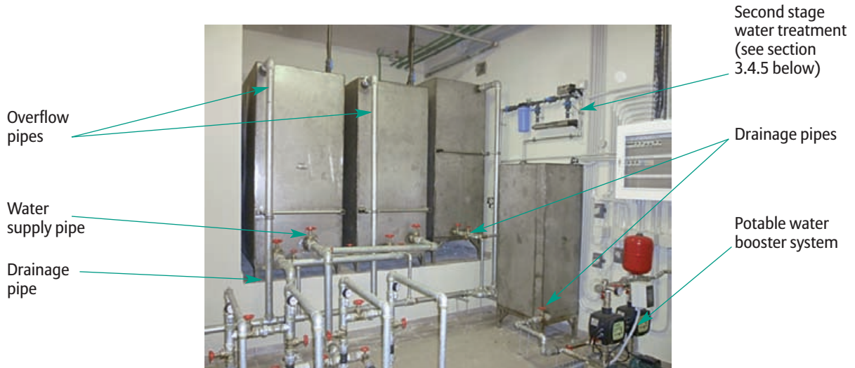
Fig. 27 Stainless Steel Tank
