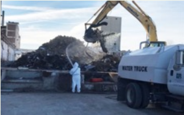
Figure 5: Manual asbestos wetting
