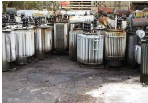
Figure 10-12 Bauchrieh Storage Site Showing Cracked Pavement and Oil Leakages
