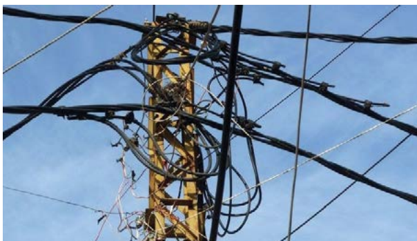
Figure 9-15 Illegal Connections to the Power Grid Photo Credit: BBC
