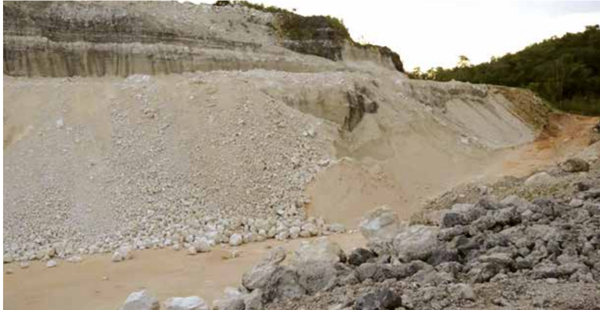
Photo 24 Group 3 Quarry: Good benching leads to more efficient & selective production, while reducing the potential for accidents
