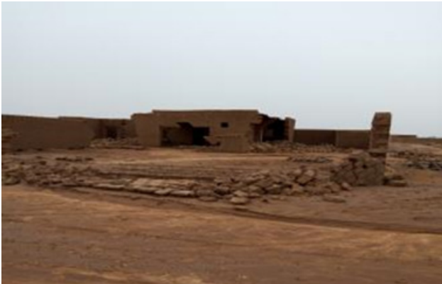
Collapsed houses in the village of Toumouga
