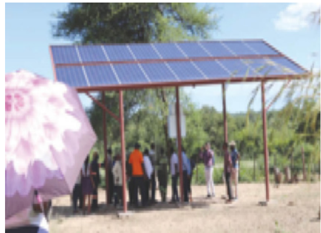
Solar water pump in Singeni Village in Nkayi District
