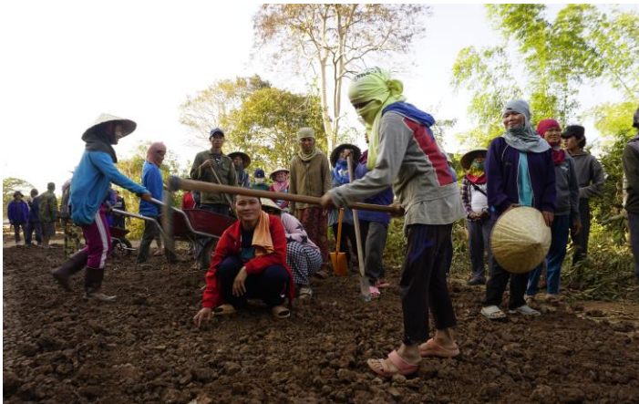
Female beneficiaries repairing a flood-ravaged road in Khammouane Province. Photo: UNDP Lao PDR/Ildiko Hamos-Sohlo
