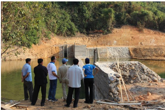
Final quality check for one of the division structures in Name Sae irrigation sub-project in Viengthong District, Bolikhamxay Province. Photo: UNDP Lao PDR/Singha Ounniyom
