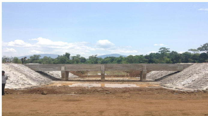
The new climate resilient drain allows flood waters to escape freely without interfering with the irrigation system. Photo: UNDP Lao PDR/Anders Poulsen
